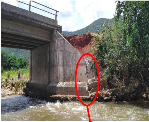
Damage to abutment wing wall
