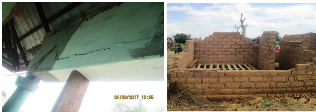
Figure 16a: Building collapse as a result of Kaputa Earthquake
