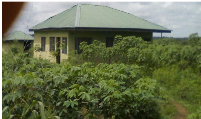
Figure 1: Abandoned and unutilized healthcare facility at Alabi village LGA (Source: Authors' Fieldwork)
