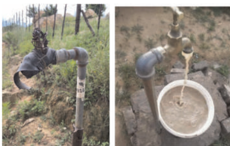
Figure 5. Poorly maintained water infrastructure.
