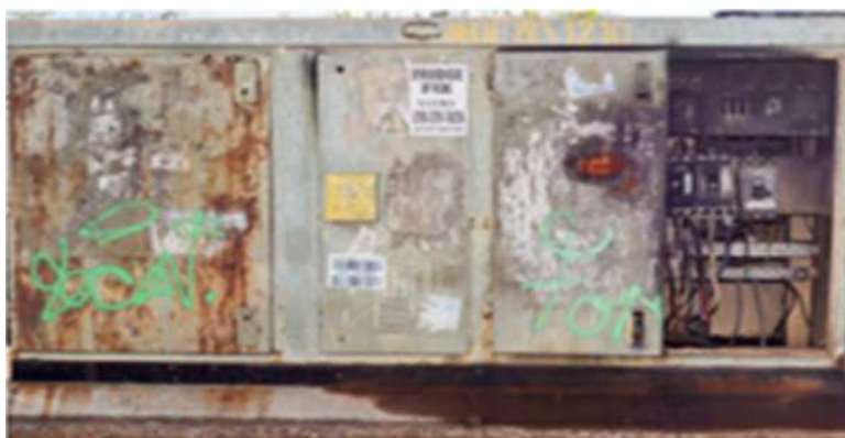
Figure 3. Status of transformers in Soweto (Author 2024).
